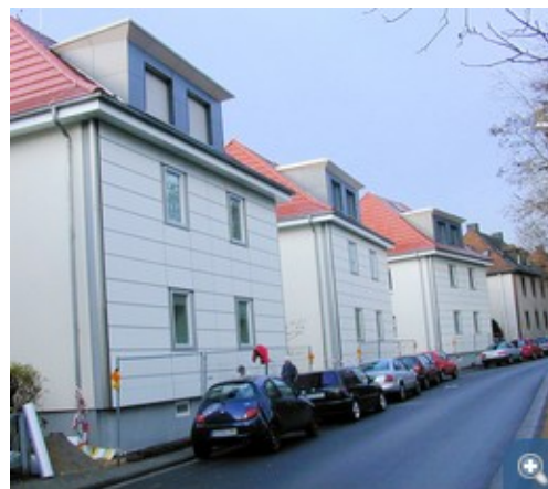
The three detached double-family houses in Wilhelmstrasse, Hofheim (Taunus) shortly after the refurbishment work was completed – and in comparison...
