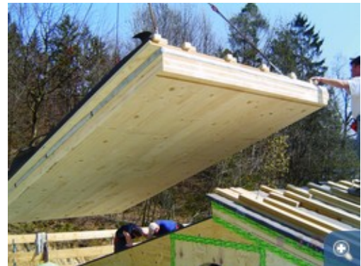
Precast roof elements with vacuum-insulation during the installation at the zero-energy-house in Voggenthal (Germany). As a grey layer the vacuum insulation is to be seen.
